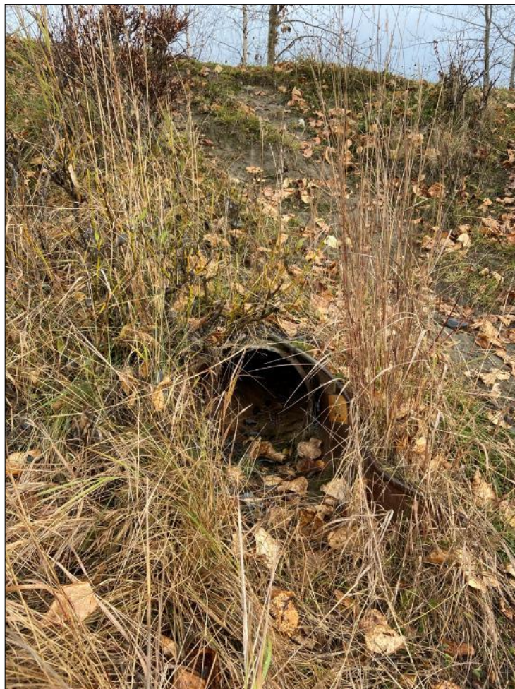
SW16. Looking northeast at west end of culvert through sewer line trail in Connors Bog
