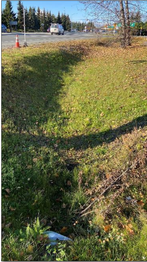
SW11. Looking northwest at culvert under Frontage Road looking northwest along Jewel Lake Road
