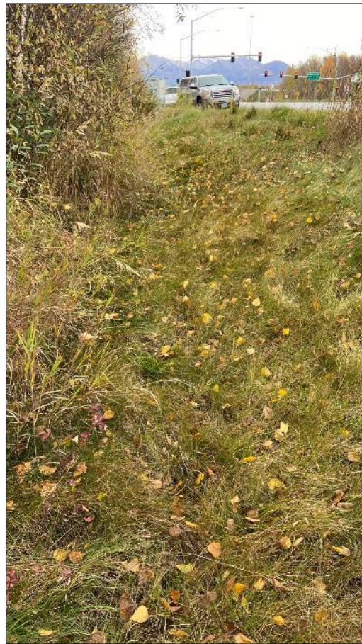
SW1. Looking east at ditch on north end of buried culvert under Raspberry Road embankment
