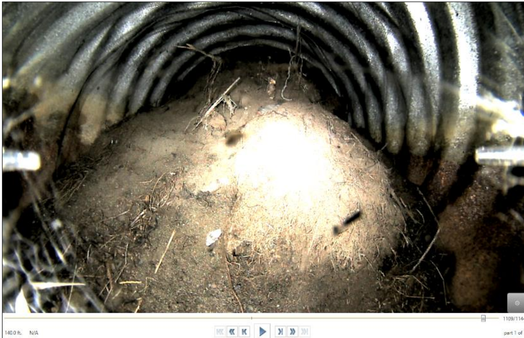
Inset 2. Blockage in Raspberry Road culvert
