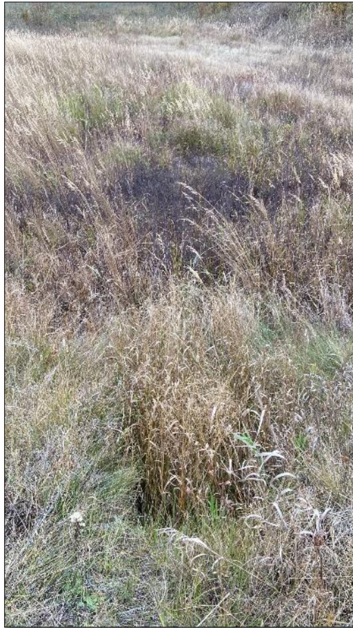
SW5. View on top of east end of culvert into Minnesota Drive offramp catch basin
