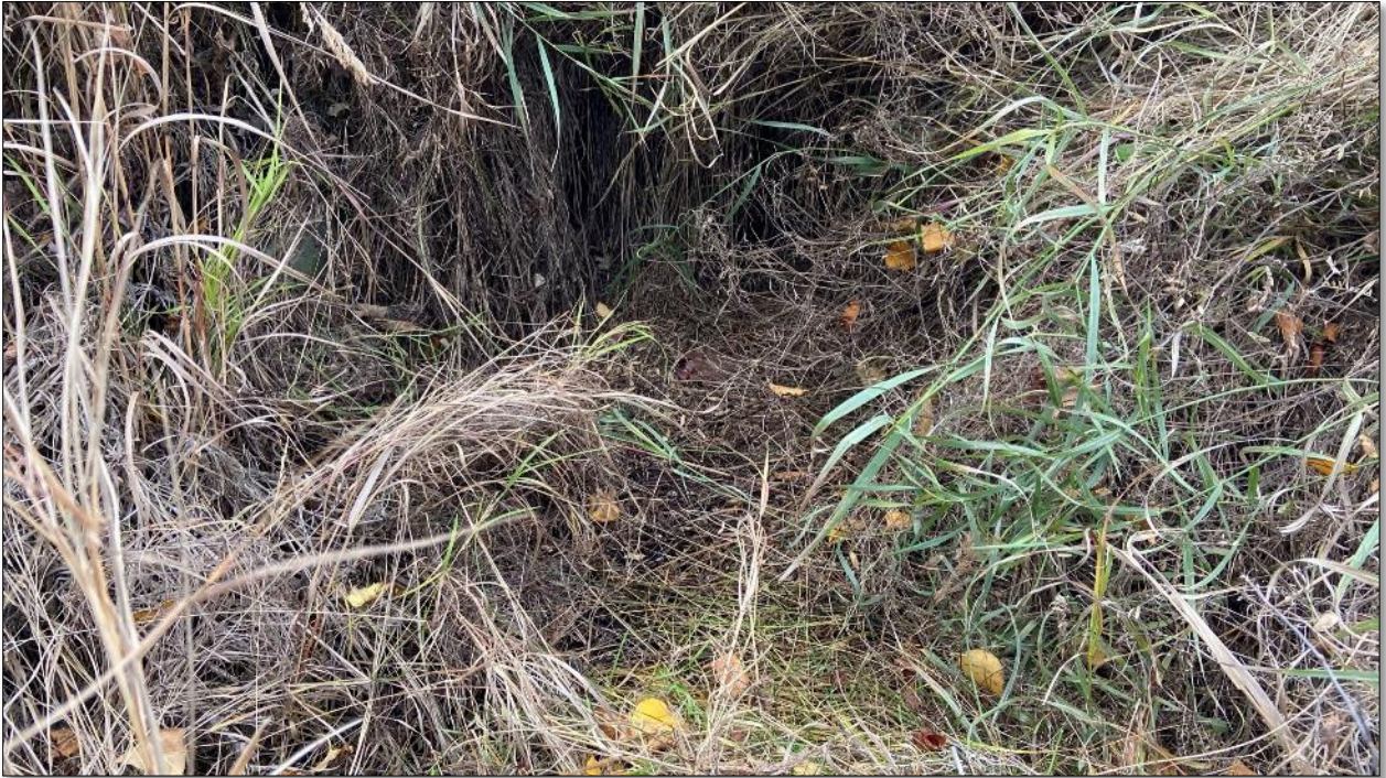
SW4. West end of culvert between Connors Bog and Minnesota offramp catch basin
