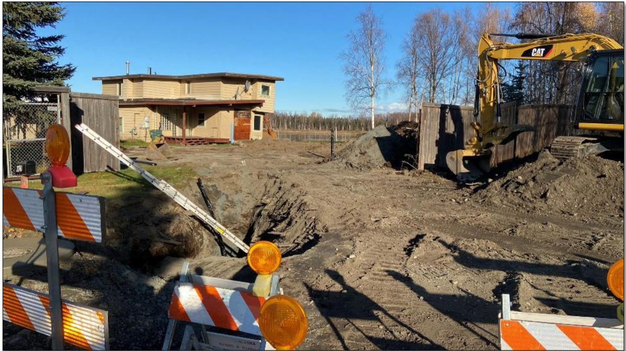
SW15. Looking northeast toward Connors Lake from point where storm drain outfall is located
